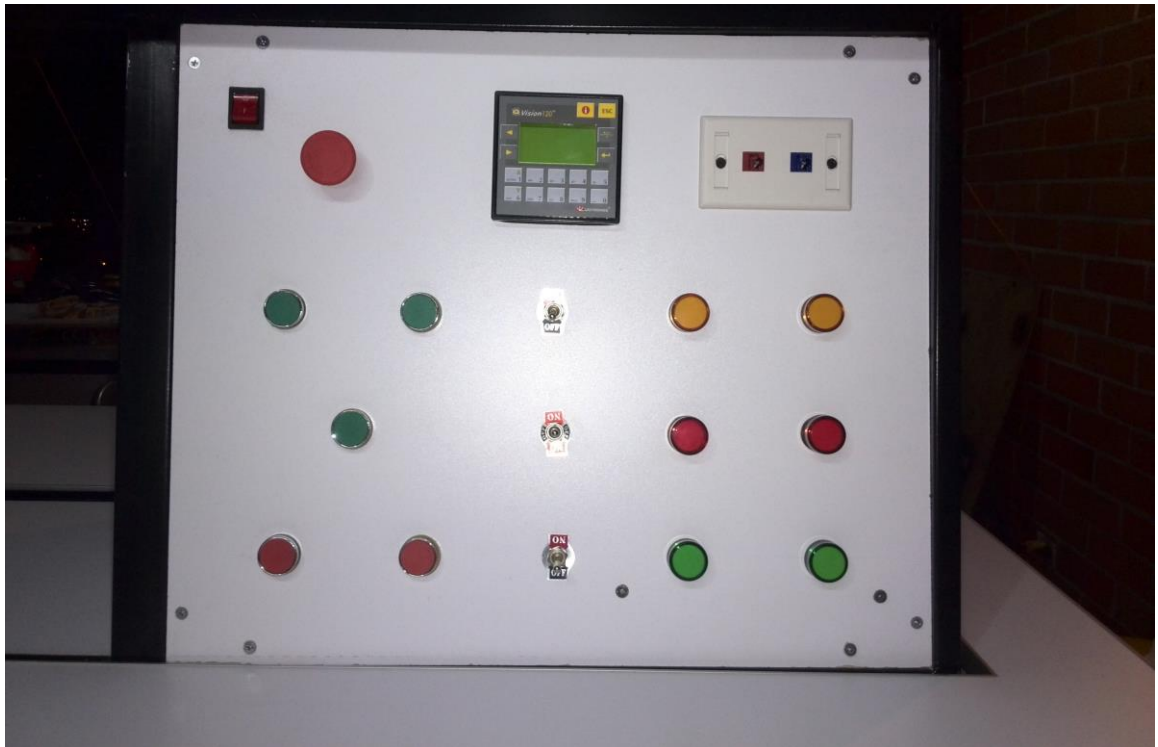
Figura 79 Panel de control del PLC
